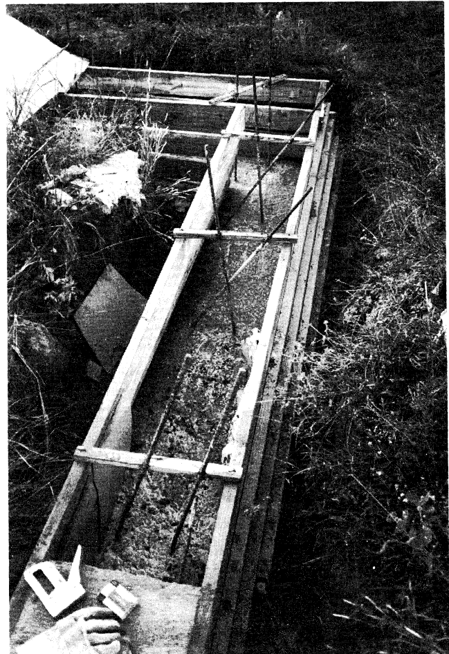
Fig. 2. Ziggurat formwork in foreground changes to the final version in the background.
